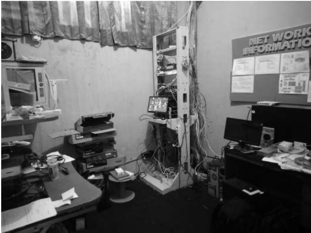
Lampiran A. Ruang ICT & Server
